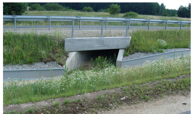
Amphibian guidance devices on the B 470 near Burk between Forchheim and Wimmelsbach
