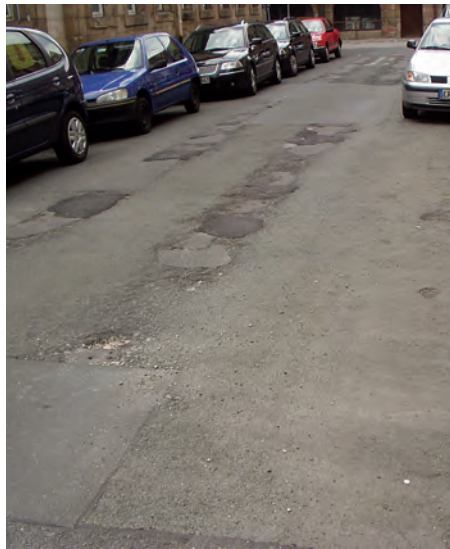
Figure 2: Road section in Erlangen requiring renovation
