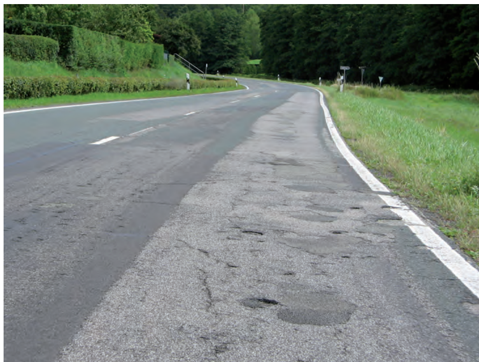
Figure 1: Road damage on a state road
