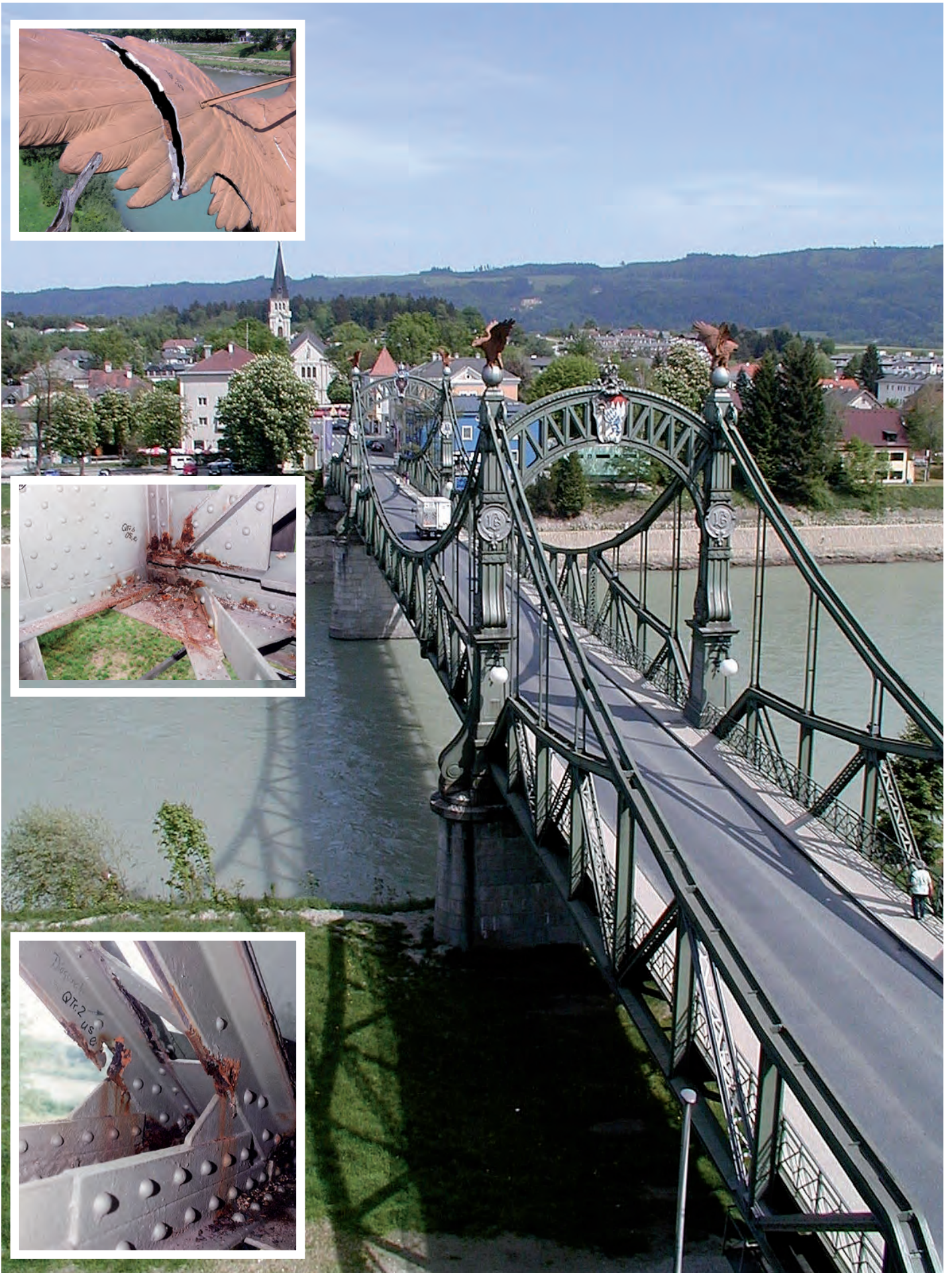
Fig. 4: State road 2103, bridge damage at the Salzach bridge in Laufen
